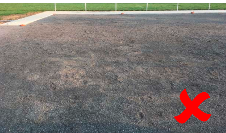
NOT LIKE THIS: gravel uneven / not sufficiently compacted.
