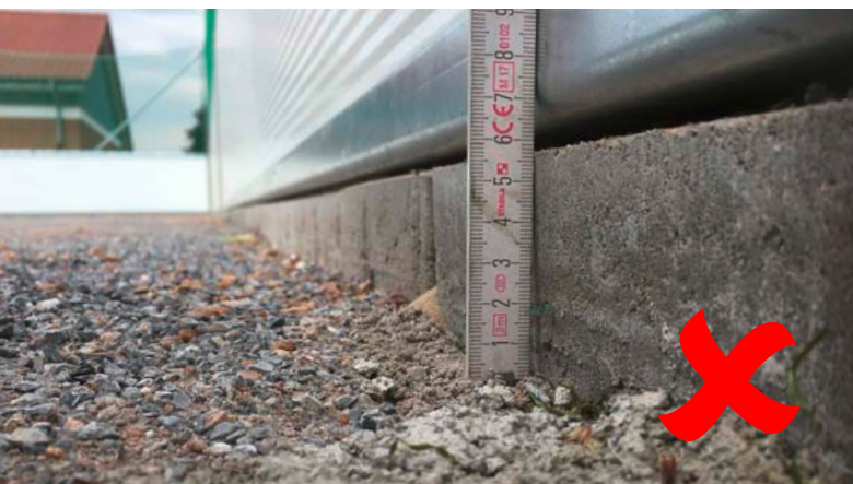
NOT LIKE THIS: installation height too high / low.
