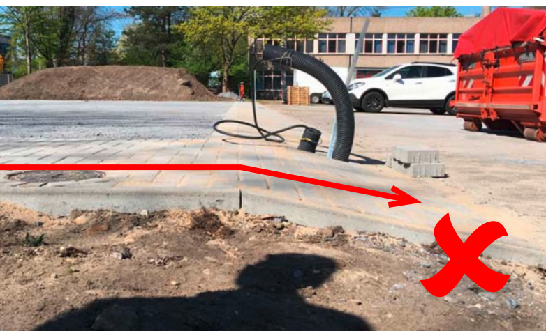
NOT LIKE THIS: surrounding paving sloping.
