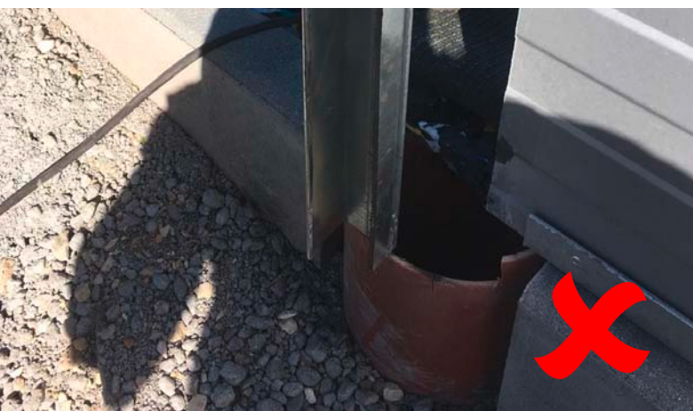
NOT LIKE THIS (if foundations): foundations placed incorrectly.
