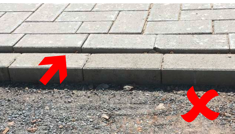
NOT LIKE THIS: paving stones not level with the curb.
