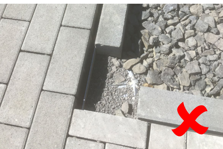
NOT LIKE THIS: foundation conduits too small or covered.
