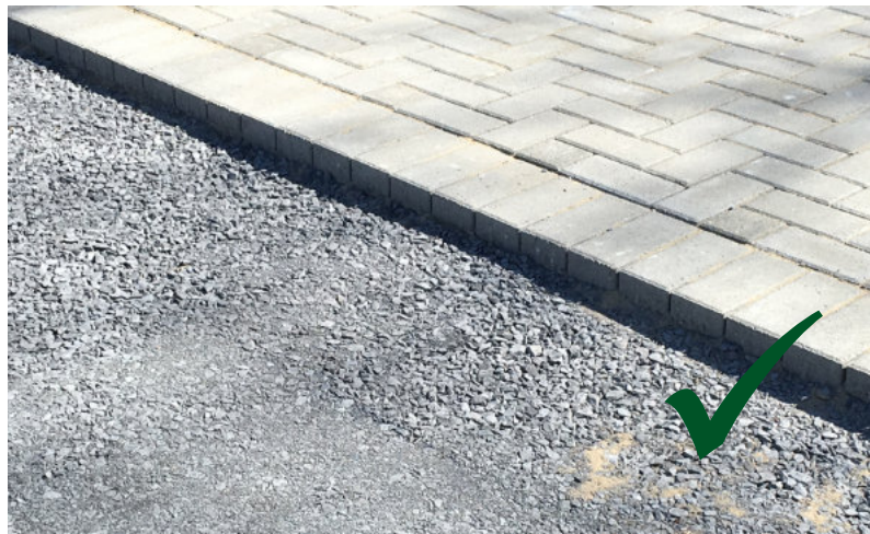
Even installation height, as specified.
