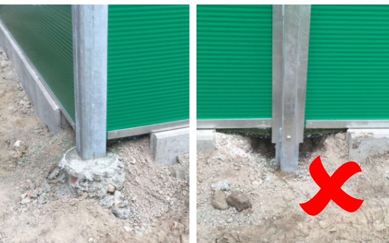
NOT LIKE THIS: curb not built right up to the conduit.
