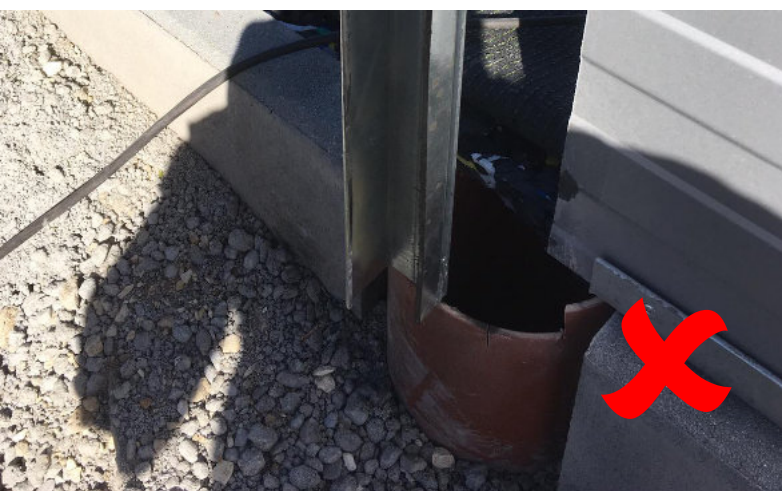
NOT LIKE THIS: foundations / conduits placed incorrectly.
