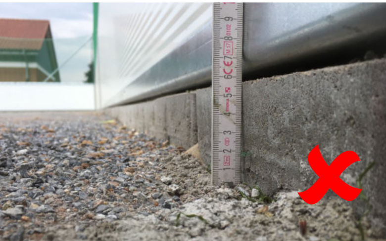
NOT LIKE THIS: installation height too high / low.
