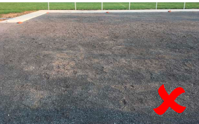
NOT LIKE THIS: gravel uneven / not sufficiently compacted.
