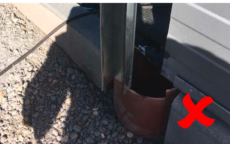
NOT LIKE THIS: foundations / conduits placed incorrectly.
