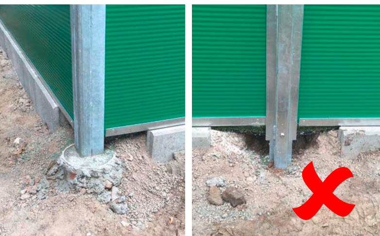
NOT LIKE THIS: curb not built right up to the conduit.
