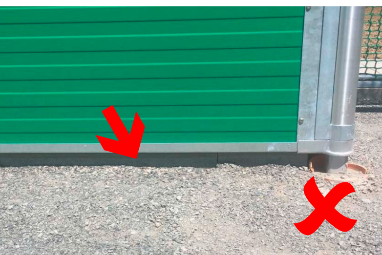
NOT LIKE THIS: curb not placed correctly (here too far out).
